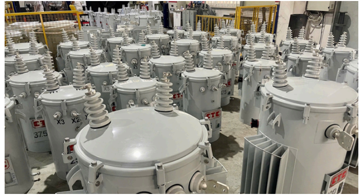
Exporter 72 transformer in PHILIPPINES
