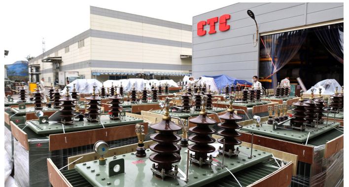
Exporter 89 transformer in LEBANON
